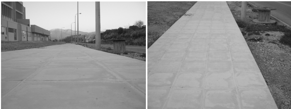
Fig. 2: Photo of the High Quality Pavement. There is no Evidence Significant Tilting or Rotation of the Plates.
