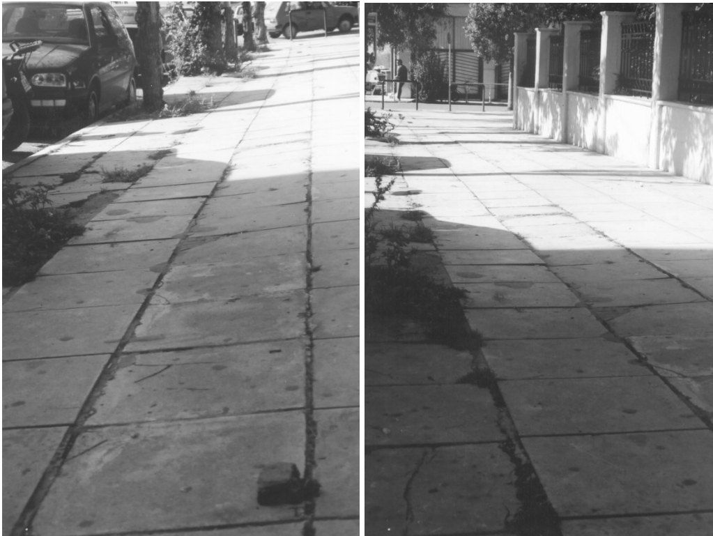
Fig. 1: The Low Quality Pavement that was chosen for the Analysis. Tilting of the Plates, Occasionally Caused by Roots of Trees are Evident.
