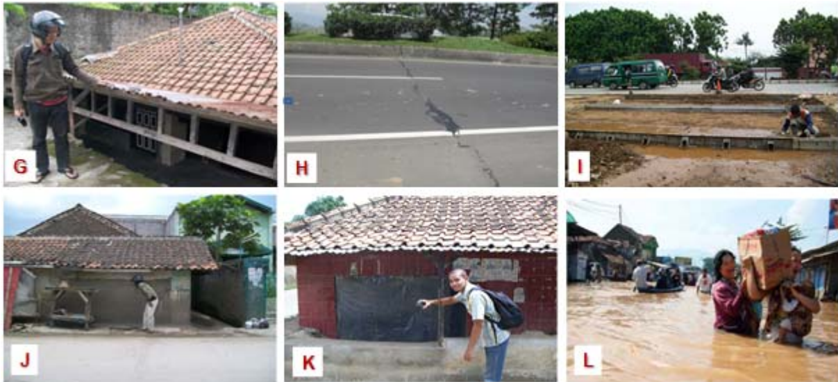
Figure 7. Examples of recent subsidence features in Bandung basin. Photos taken by Irwan Gumilar in 2010. In this Figure G: Subsided house in the Dayeuh Kolot area (around DHYK GPS stations); H: Highway cracking in the southern Cimahi area (around CMHI GPS station); I: Uplifting of the road due to subsidence in the Gedebage area (around GDBG GPS station); J: Subsided house in the Gedebage area (around GDBG GPS station); K: Subsided house in the southern Cimahi area (around CMHI GPS station); L: Flooding in Dayeuh Kolot area (around DHYK GPS station).
