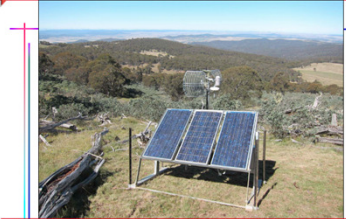
The LocatNet "receivers" deployed on hilltops for these trials are powered by simple solar panel arrays. The antennas are mounted on a basic stand. This will on Mt. Roberts transmits only 20 watts for synchronization with other LocatNets over 40-50 km away.
