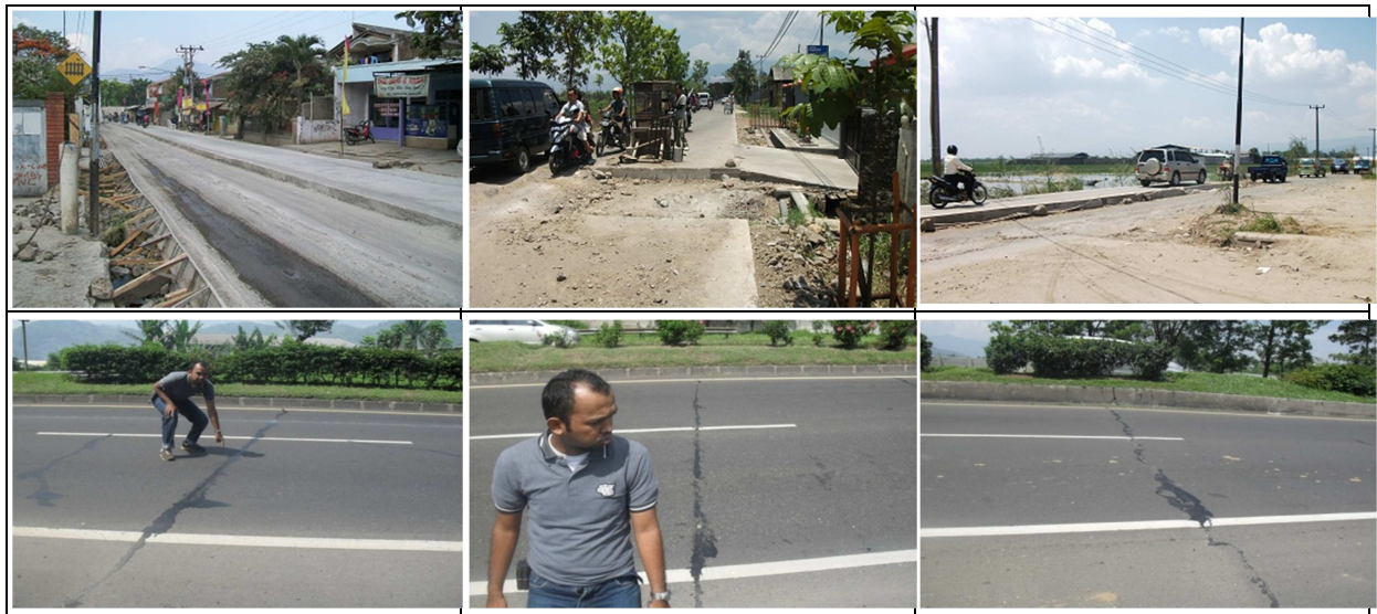
Figure 10. Impact of land subsidence on cracking of road and highway road in Bandung Basin
