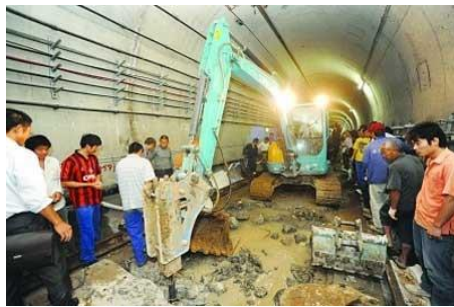
2011.08.22 Subway tunnel damage Nanjing, China
