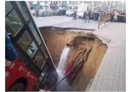
2020.01.13 Road surface collapse Xining, Qinghai, China 4 people died
