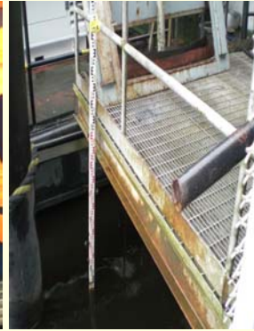
Tide Gauge Installation at the project area.
