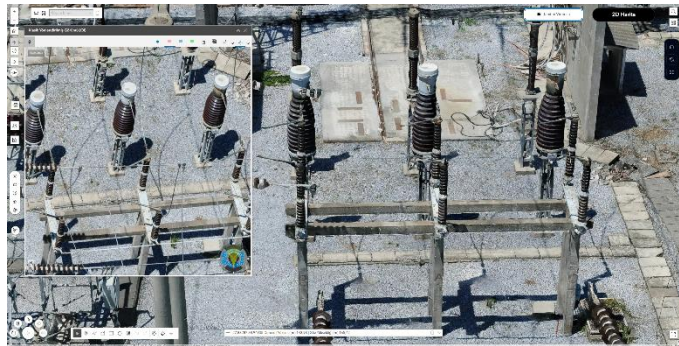
Figure 4: An example of oriented imagery from the substation
