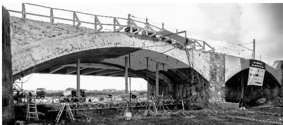
Figure 1. Side view from West of the arch 4 of the historic masonry arch bridge. The whitewashed area indicates the area of the direct influence of the load application. On the bridge: four hydraulic cylinders for the load application (Paffenholz et al., 2018a).
